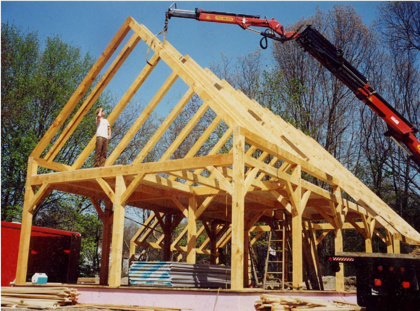
above: Construction of Center Street Studio at its present location in Milton, MA in 2001. The Shelter Institute from Woolwich, Maine built the studio in traditional post-and-beam construction.
